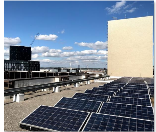
Solar installation at Portsmouth City Council
