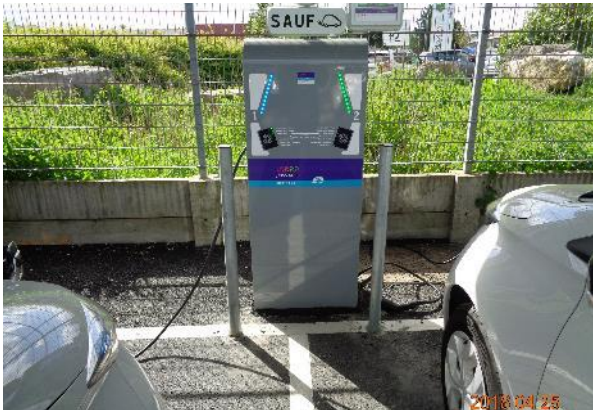
Electrical charging station DIVA SP 3-22KVA (Total EV)
