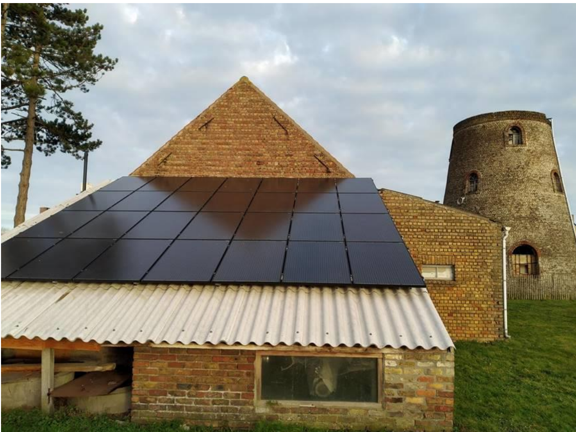
Figure 3: Installed PV system on the renovated roof. The Groenhage Mill tower (Groenhagemolen) can be seen in the background.
